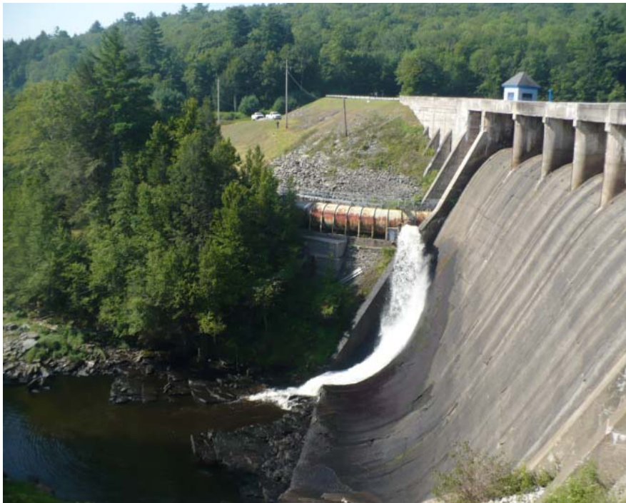
Rio Dam Project, Forestburgh, New York (2014-ongoing) Computational Fluid Dynamic (CFD) Flow 3D analysis
